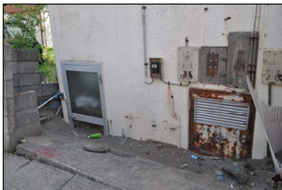
Settlement of building resulting from ground liquefaction in Japan
