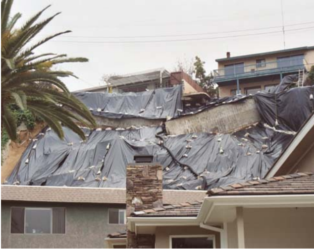
Slope and retaining wall failure in Culver City
