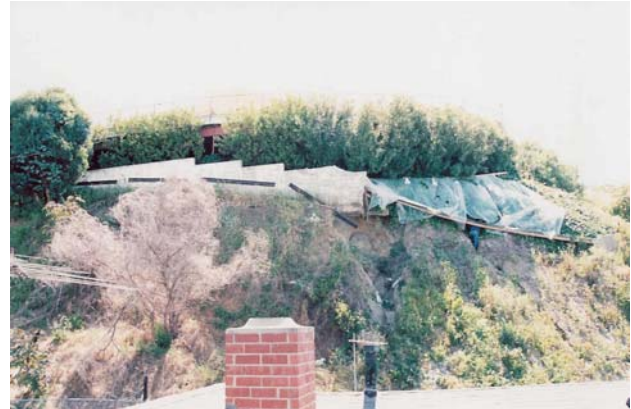
Collapsed retaining wall damages home below
