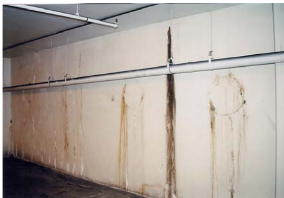
Seepage through wall (inadequate waterproofing)
