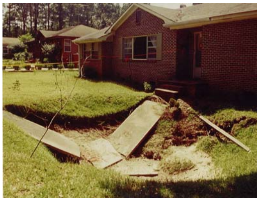
Sinkhole in the front yard of a residence
