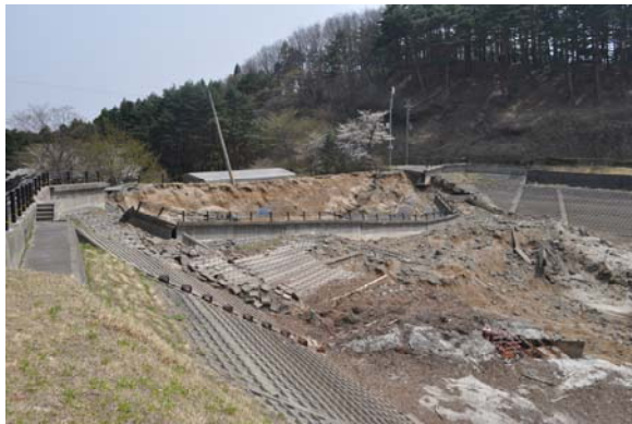
Figure 2 Photograph of the failed Fujinuma Saddle Dam
