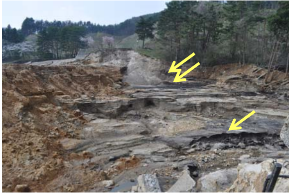
Figure 1 Photograph of the breached Fujinuma Main Dam (the arrows point to a layer of dark and organic residual soil)
