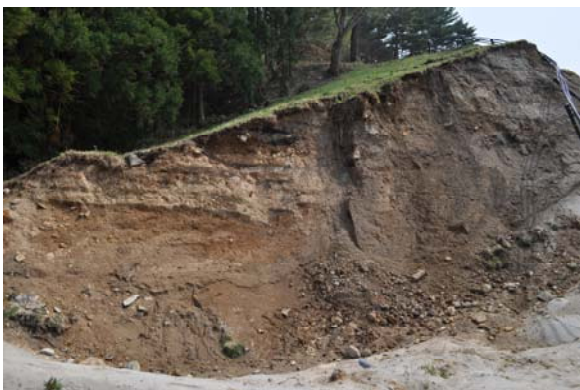
Figure 3 Photograph of a near vertical section of the Fujinuma Main Dam breach (looking South).
